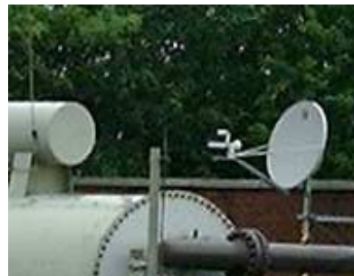
Remote VSAT equipment.
